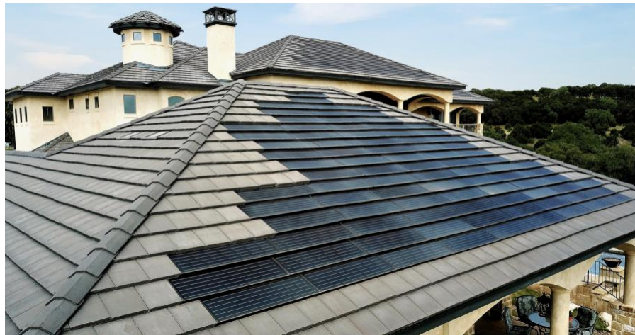
Example above of a "Patchwork" Solar Tile installation that is NOT allowed.
